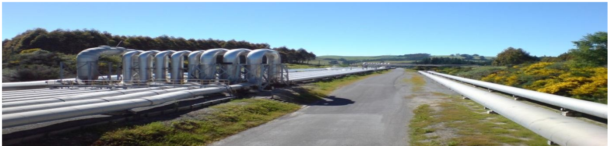
Fig No .02 Steam pipelines leading from a steamfield leading from a steam field near Lake Taupo to the geothermal power plant at Wairakei Region of Waikarto
